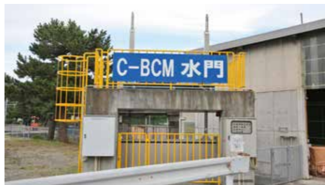
Sluice gates for tsunami countermeasures
